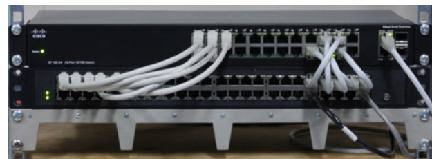
Figure 6: Ethernet switch and sync pulse injector.
